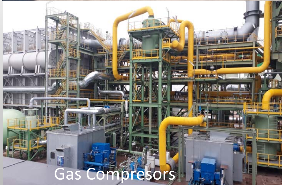
Reformer & Heat Recovery
